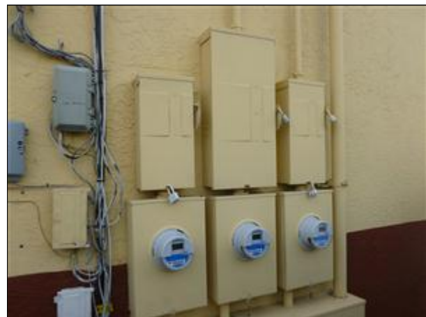
Meters and Disconnects
