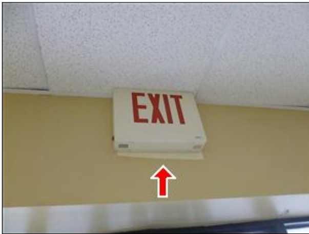
Non-Lit Exit Light - Suite 1
