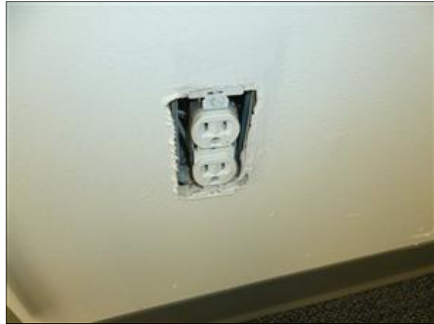
Missing Trim Plate - Suite 3
