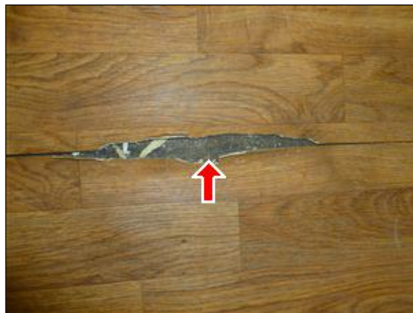
Damaged Flooring - Suite 2
