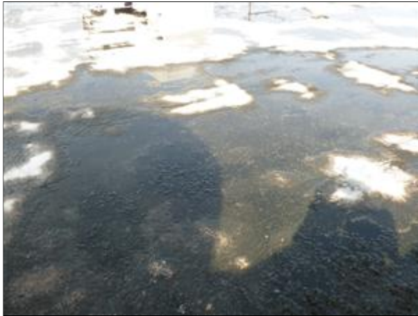
Roof Showing Standing Water
