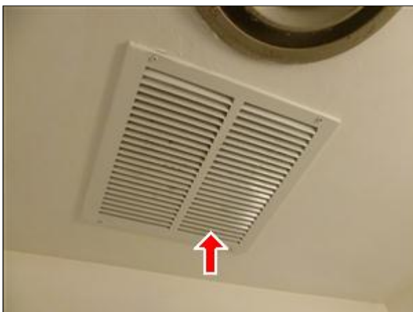
Bathroom Vent - Suite 3
