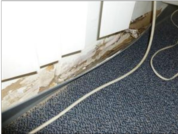
Damaged Floor Base - Suite 2
