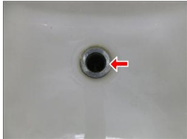
Missing Drain - Suite 2
