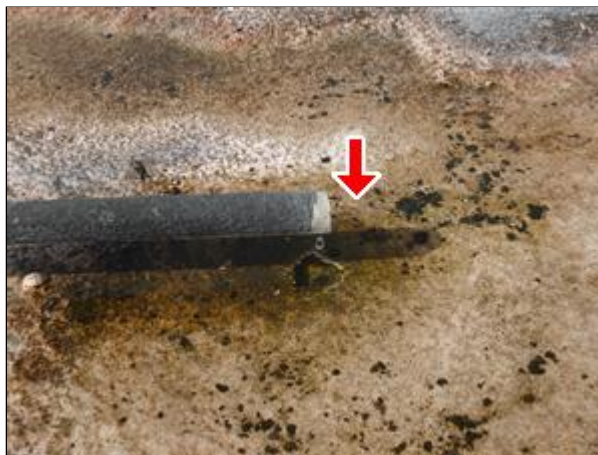
Broken AC Drain - Roof
