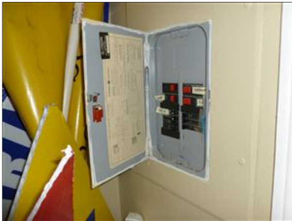
Electrical Panel - Suite 1
