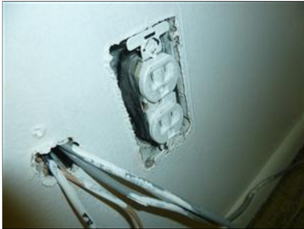
Missing Trim Plate - Suite 3
