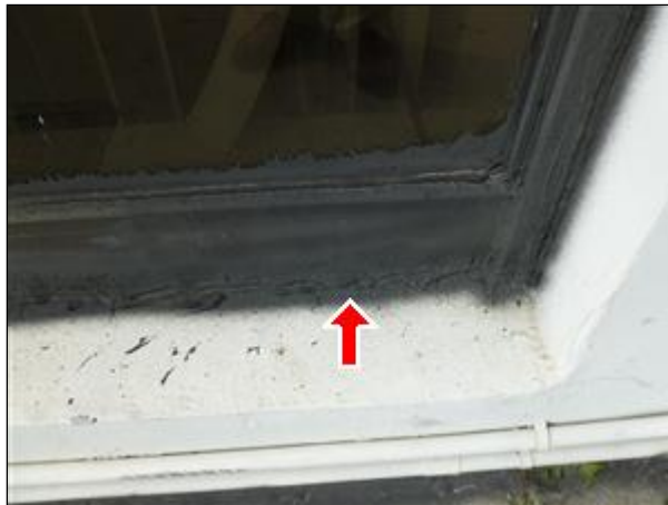
Deteriorated Window - Suite 2
