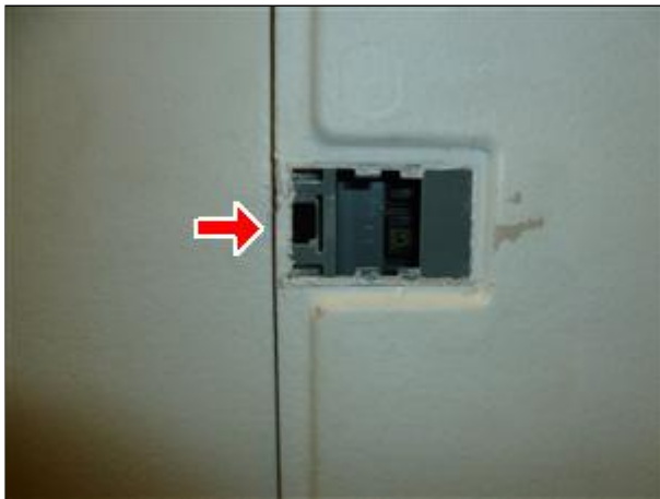
Damaged Panel Cover - Suite 2
