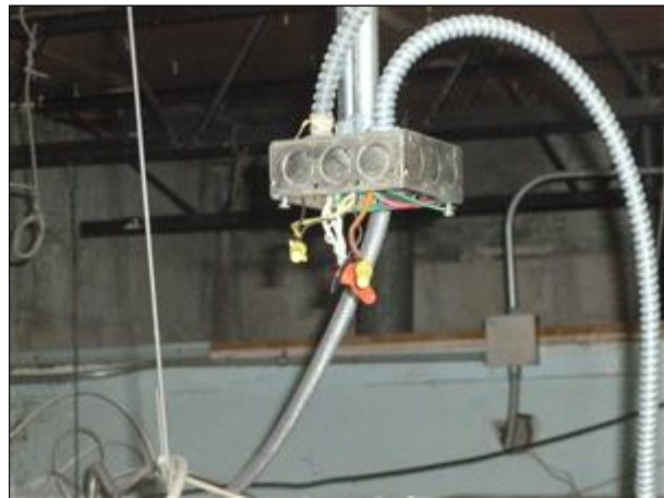
Open Junction Box - Suite 3
