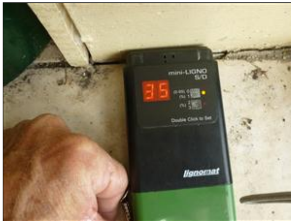
Front Entry Moisture - Suite 1
