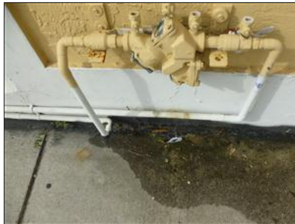
Leaking Back Flow Preventer - East Elevation
