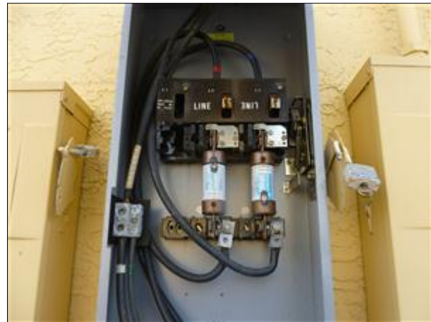
Electrical Disconnect - Suite 2
