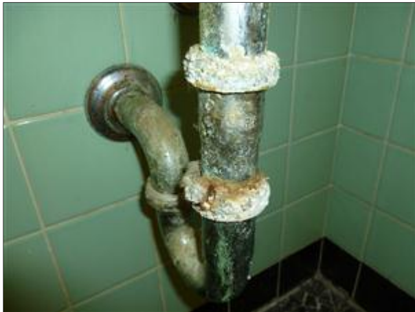
Corroded Drain - Suite 3
