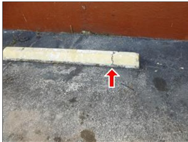
Damaged Car Stop
