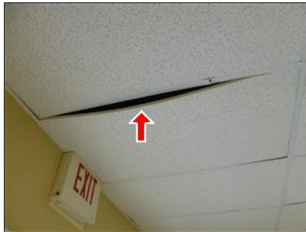
Damaged Ceiling - Suite 1
