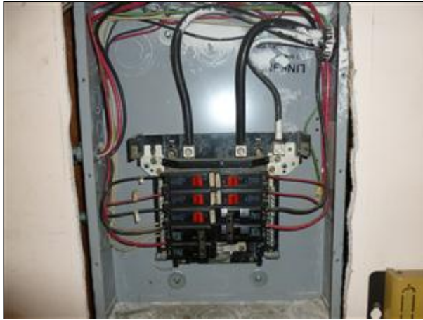
Electrical Panel - Suite 3
